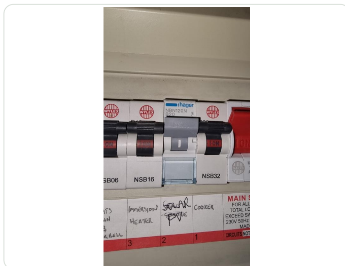
AC breaker: ON
