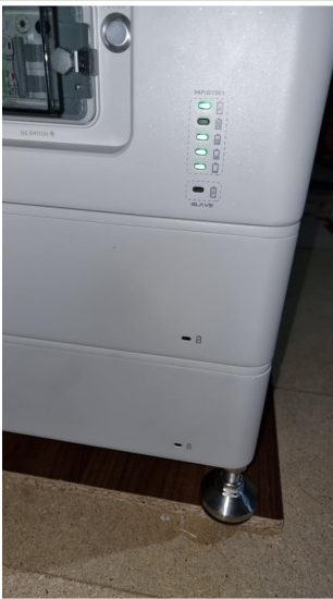
Battery modules showing green
