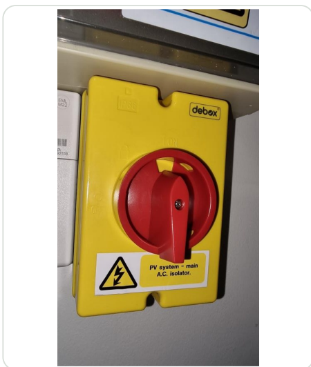
AC isolator: ON
