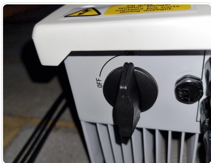
PV DC isolator: ON
