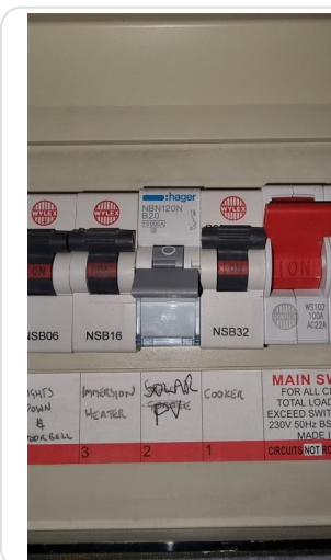
AC breaker: OFF
