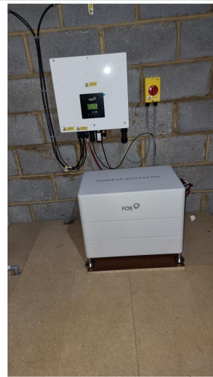
Completed expanded battery stack
