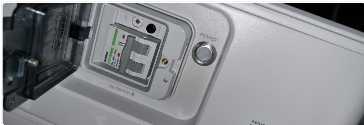
Battery power and DC breaker: OFF
