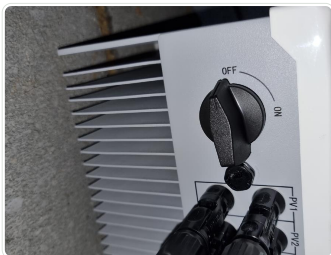
PV DC isolator: OFF
