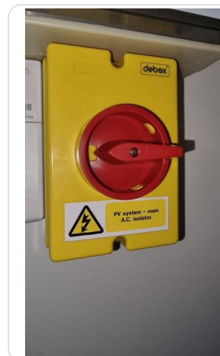
AC isolator: OFF
