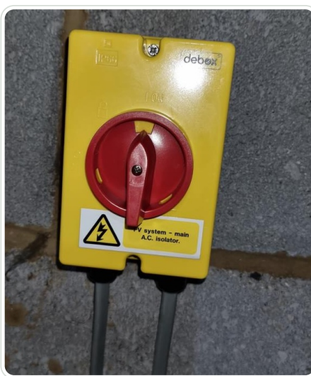
Additional isolator: ON
